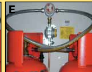
Picture shows a Truma regulator upgraded to an Auto changeover with a 01-1755 and using two propane 0.75 meter Stainless hoses. Note how the hoses cross preventing unnecessary kinking and twisting.
