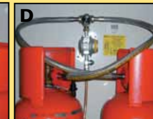
Picture shows a Truma regulator upgraded to a manual changeover with a 01-1630 and using two propane 0.75 meter Stainless hoses. Note how the hoses cross preventing unnecessary kinking and twisting.
